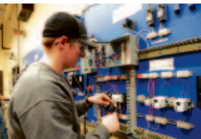
Jonathon Aurand of Selinsgrove wires a reversing motor control circuit in the Electrical Systems Technology program at SUN Tech.
