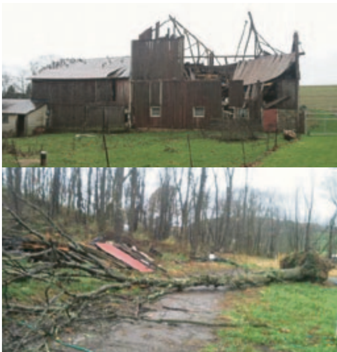
Top: Barn in Union County damaged by storm. Middle: More storm damage in Union County. Bottom: Storm damage in Snyder County.
